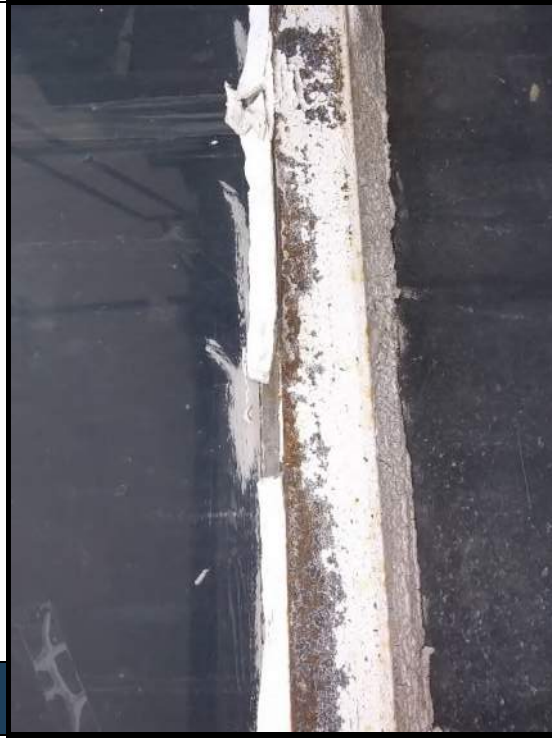
4 Window glazing tested positive for asbestos (2% chrysotile).
