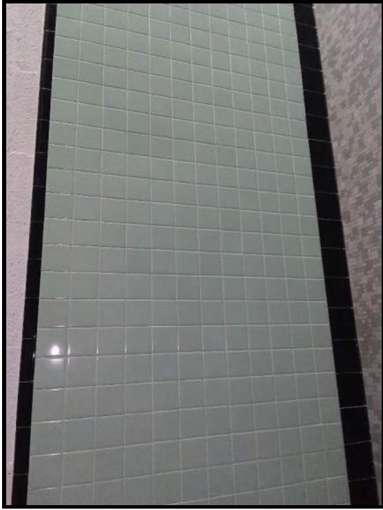
10 Green and black ceramic tile in men's restroom tested positive for lead based paint (5.40-19.90 mg/cm 2 ).
