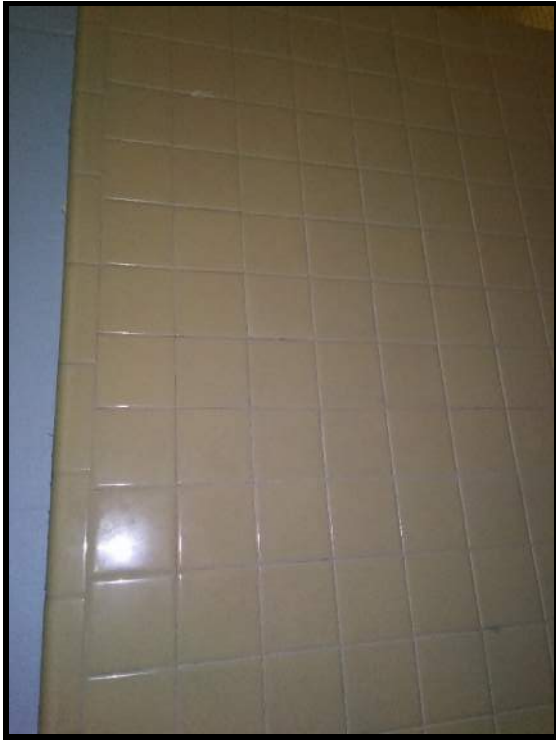
9 Yellow ceramic tile in men's restroom tested positive for lead-based paint (7.70 mg/cm 2 ).
